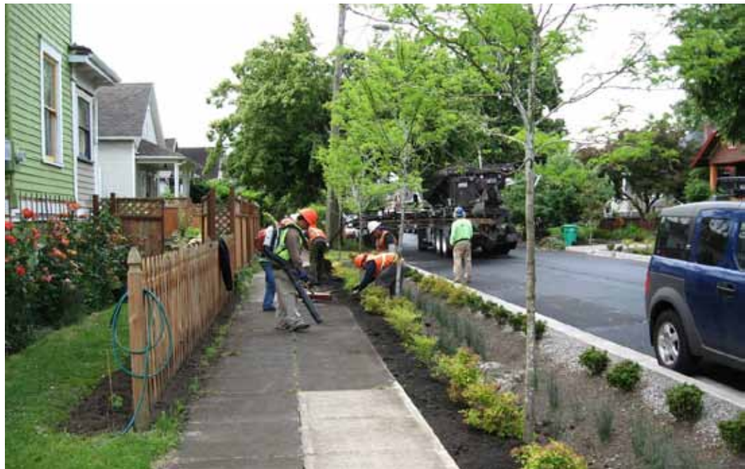
Greenstreet projects, such as this one for Portland's "Tabor to the River", can cost up to 40% less than the traditional "grey" street upgrade. Photo Portland Bureau of Environmental Services
